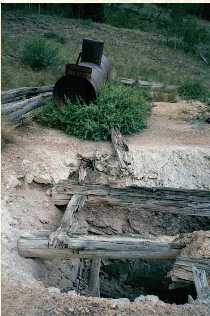
Lying in wait. Old mines present structural hazards such as the danger of collapse or accidental falls.
